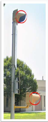
Signs not located at beginning/end of school zone on East Putnam and neither the sign nor the flashing lights can be read from Old Church Road approach
